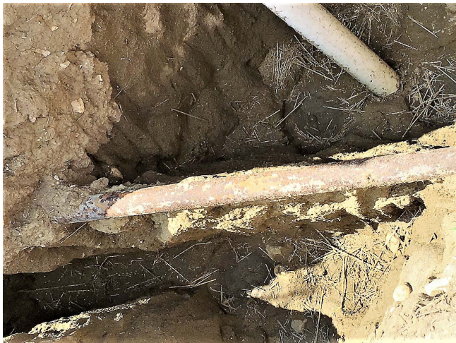
Figure 1. A 2 in. steel oil pipeline in the Bakken Formation of North Dakota, USA, with mostly degraded external coating (a second pipeline is directly underneath).
