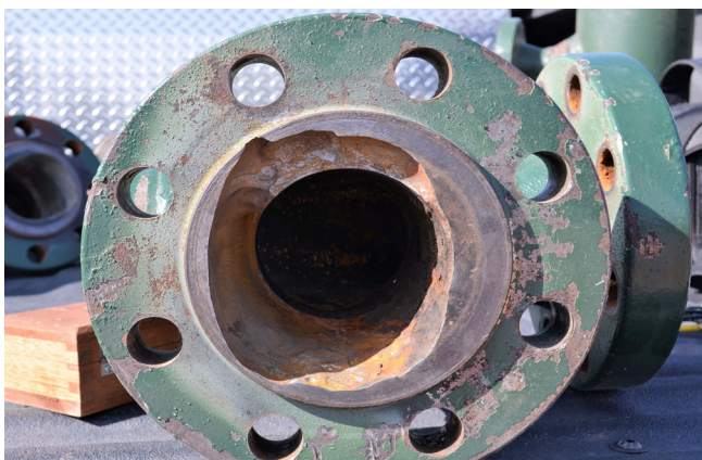
Figure 2. A corroded 8 in. flange face on emulsion pipeline at isolation kit, with CP current transfer through produced water fraction (combination of emulsion water content and stray CP current).
