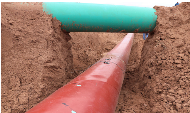
Figure 3. A foreign pipeline (green coating) crossing the client's pipeline. Light-coloured spots on the red line are coating damage from CP interference.
