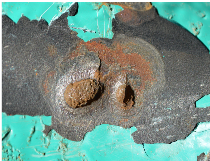
Figure 1. A 0.3 in. wall, 6 in. elbow with field coating. Pits were not evident until the removal of never-adhered (but intact) field-applied coating in the shop; corrosion product still partially fills both pits, one of which was 0.24 in. deep (80% wall loss). Note that coating had not cured before backfilling began. A through-wall external corrosion pit was found several inches to the right, at a girth weld.
