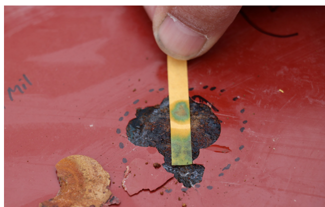
Figure 4. In-between dig and exposed pipeline metal with acidic conditions.
